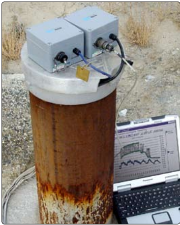
● Two Single-Channel, LC-2 Dataloggers monitoring Vibrating Wire Piezometers.
