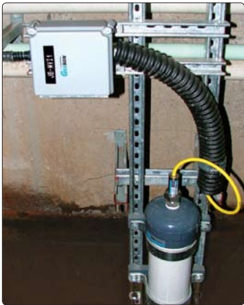
● Single-Channel, LC-2 Datalogger, used in conjunction with Model 4675LV Vibrating Wire Weir Monitor, to measure seepage in dam gallery.
